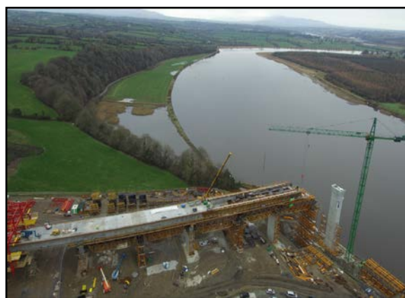
Barrow Bridge at Pink Rock – central deck cast and struck for spans 1 & 2, false work removed from span 1.
