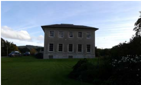
Kilrush House – Removal of defective plaster and replacement with appropriate lime plaster
