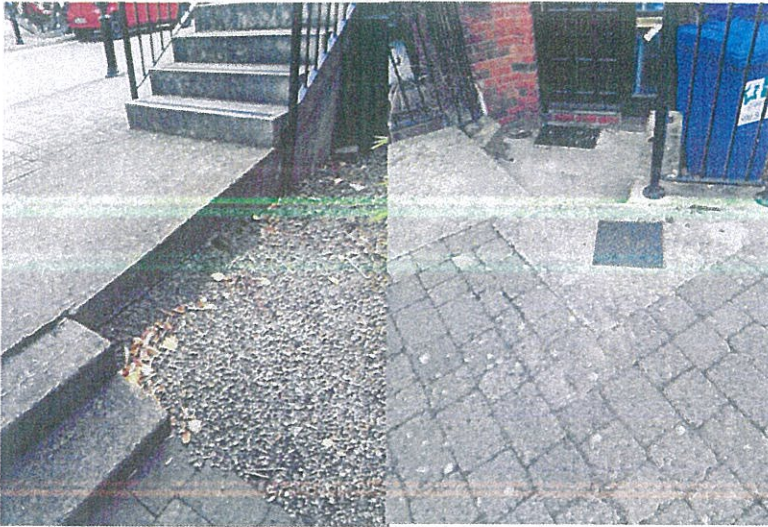
View of steps down, from below. View of steps down, from footpath.
