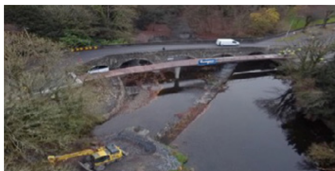
Overview with the new Castlecomer Footbridge in position (just after the bridge lift)
