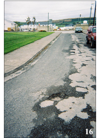
Photo 16: Poor road surface associated with housing development at 'The Orchard'.
